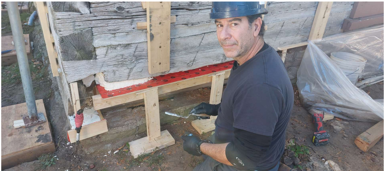
Top: Scadding Cabin exterior as seen during repairs, October 2023. Bottom: Bruno DiSalvo of J. D. Strachan Construction applying epoxy to limit rot before installing the new log. Photos: David Rayment.
