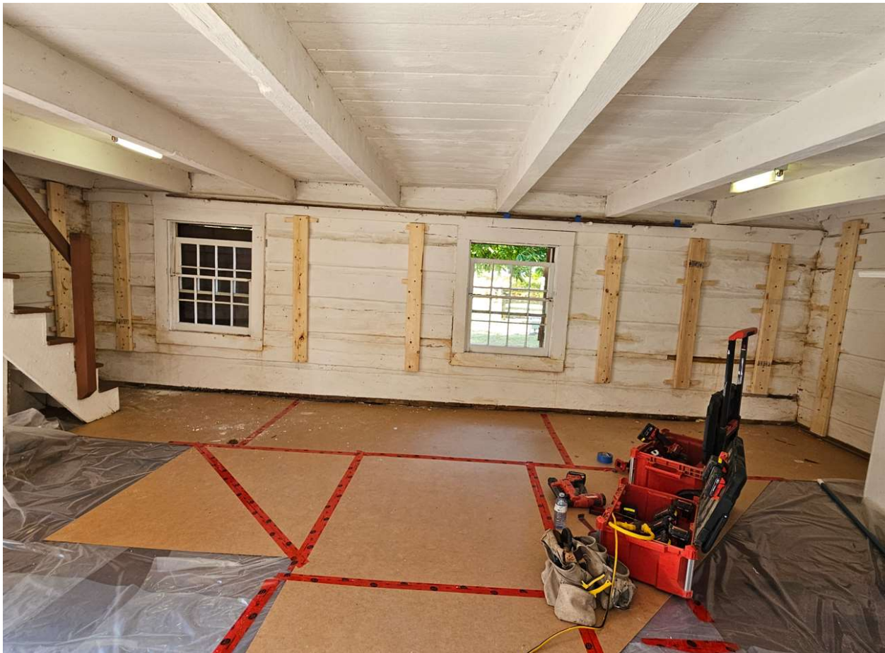
Above: Scadding Cabin interior as seen during repairs, October 2023. Photo: Kayoko Smith.
